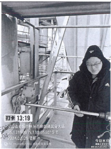
矿渣微粉1#成品仓废气排气筒出口
